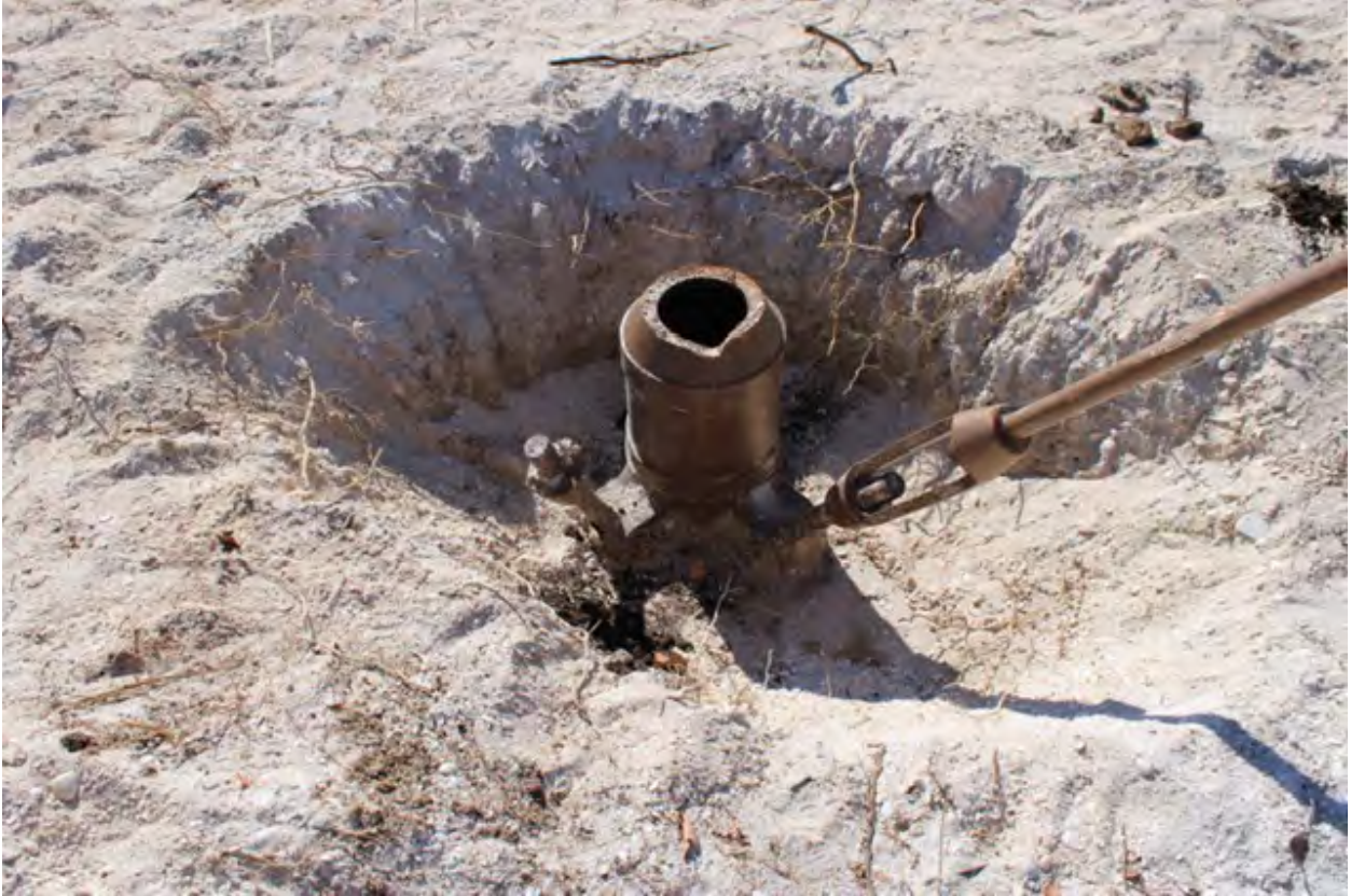
(4) The main support columns at the northwest corner of the tower indicating how it was sheared off at its connection point.
